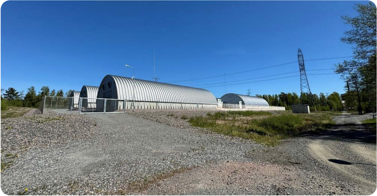
Figure 9. Current battery energy storage system in the area.
