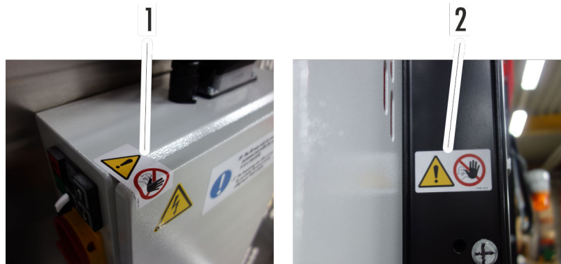
Fig. 7: Seal on control cabinet and overload
