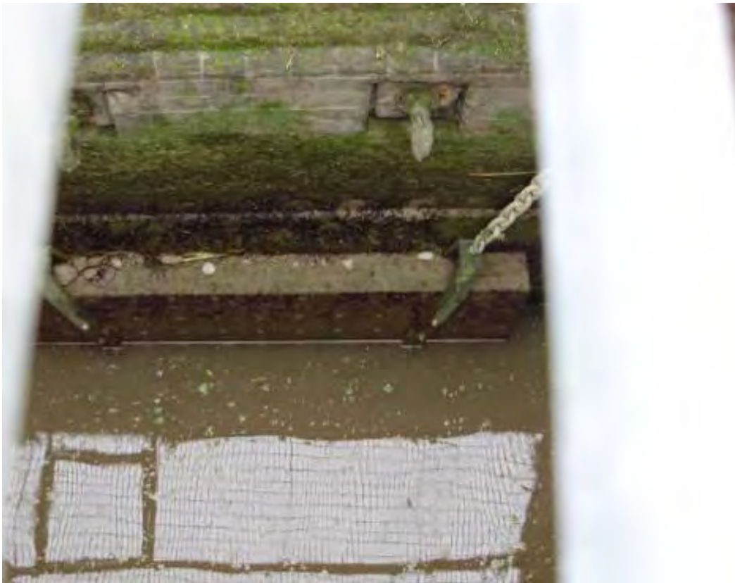
Plates 16.19 and 16.20: Great Arch Sluice Inspection chamber at low tide (top photo) and high tide (bottom photo).
