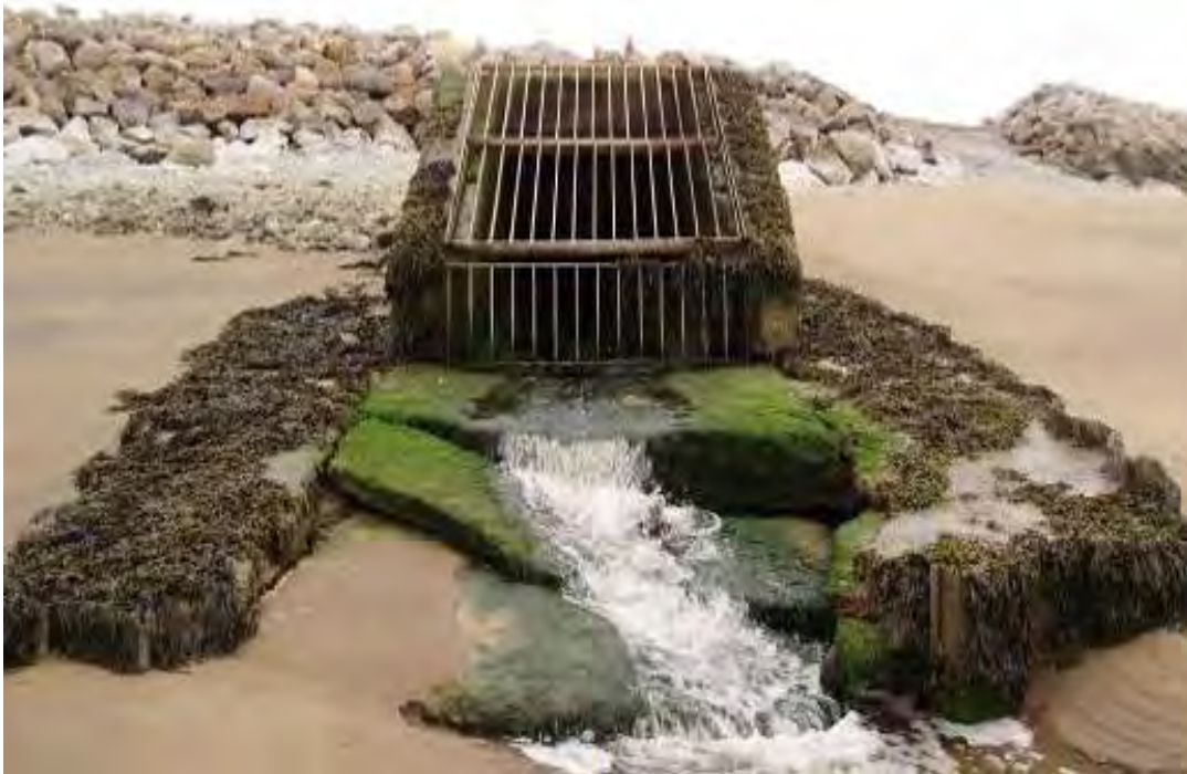
Plates 16.17 and 16.18: Photographs of Great Arch Sluice upstream face (top photo) and outfall on the foreshore (bottom photo).
