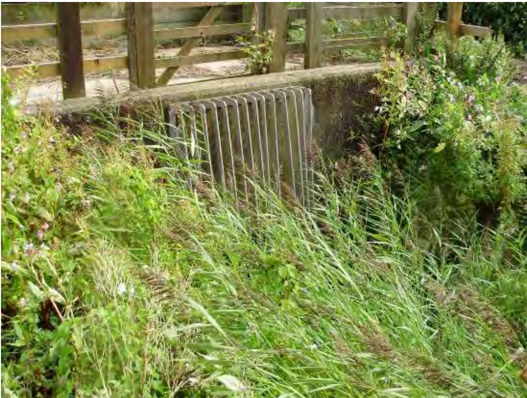
Plates 16.21 and 16.22: Photographs of Rhyne East looking towards Cole Lane Sluice (top photo) and Cole Lane Sluice (bottom photo).
