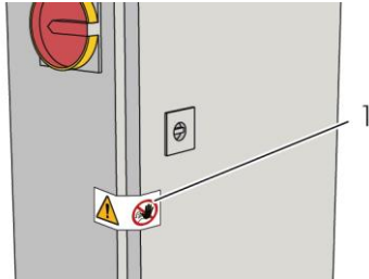
Fig. 62: Seal on switch cabinet
